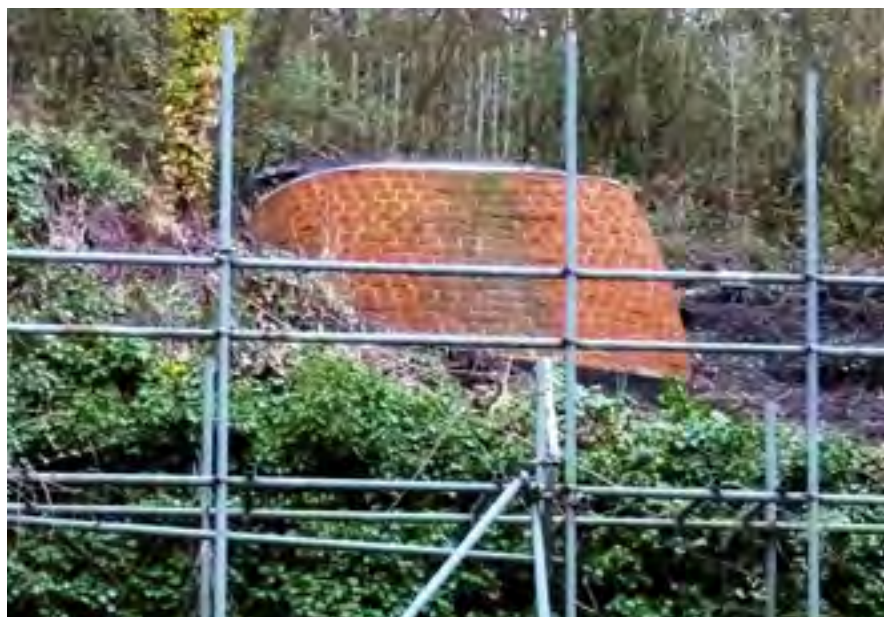
Brockham lime kiln, which was rebuilt for Surrey Wildlife Trust to protect local bat colonies
