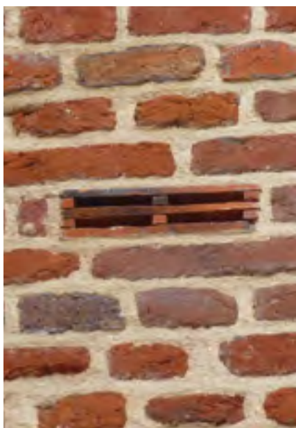
A tile slip bat access vent
